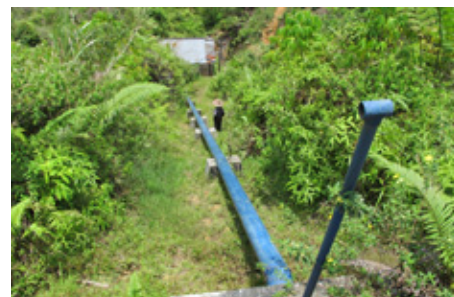
The penstock and powerhouse of the 11 kW hydro plant at Palanggaran. The pipe in the foreground is for pressure release.
