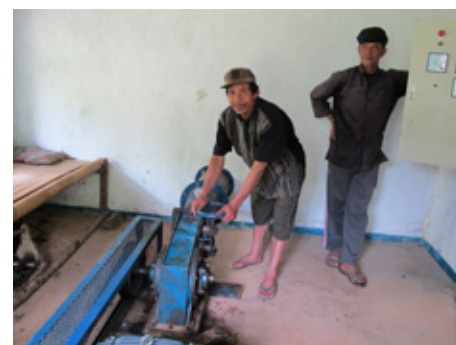
The hydro operator at Palanggaran starts up the plant in the afternoon by opening the inlet valve to the turbine.
