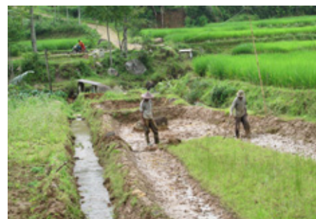
Constructing a fishpond to make use of the water coming out of the Cicimet hydro plant.
