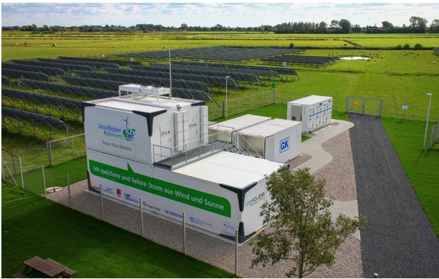
© E.ON. Hybrid storage system combines a redox flow and a lithium ion battery to provide high energy and high power.
